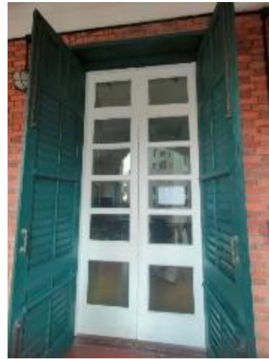
Fig. 61. Laboratory rooms with louvred shutter windows toward the verandahs. The tilt rods of the shutters control the level of openness. Door stays to fix the louvred shutter aside to allow no blockage of natural light while full open is necessary.
